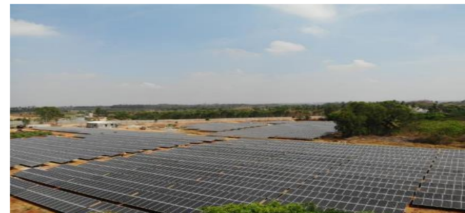
Solar Panels at HRGRDC, Bengaluru
