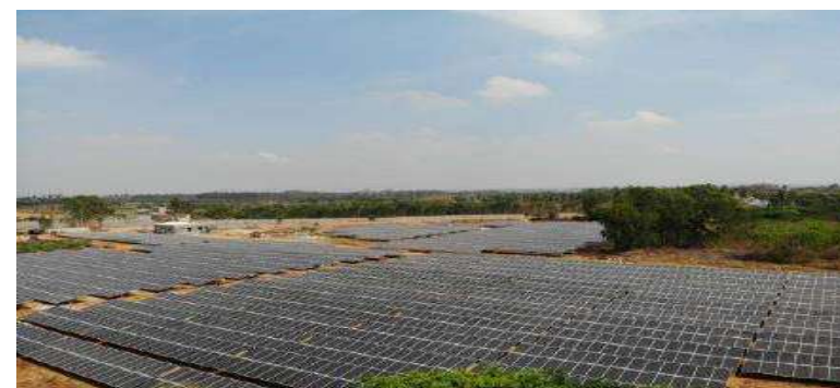
Solar Panels at HRGRDC, Bengaluru
