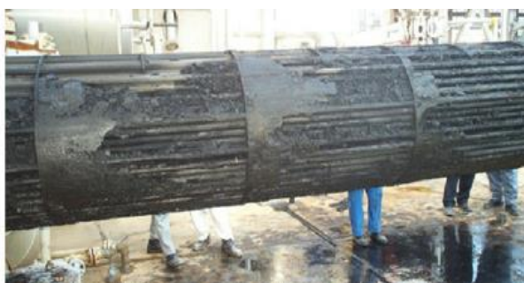
Fig.1: Fouled heat exchanger
