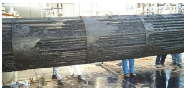
Fig.1: Fouled heat exchanger
