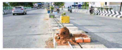
A view of the damaged and dried-out ornamental plants on Thiruvanaikovil bridge median in Tiruchy district | M K ASHOK KUMAR
