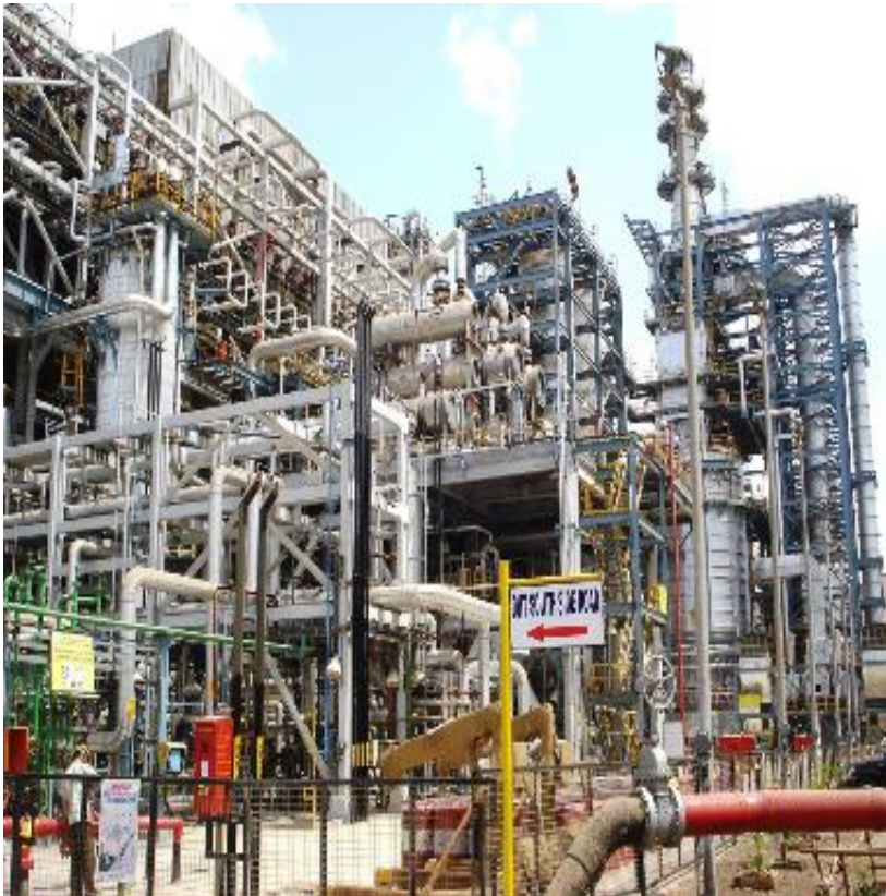
Mumbai Refinery - 1.76 MMTPA
